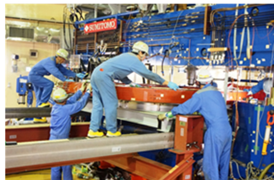
Fig. 2. Pictures of the main coil replacement work. Removing the vacuum chamber (upper) and the upper main coil (lower) from the magnet yoke.
