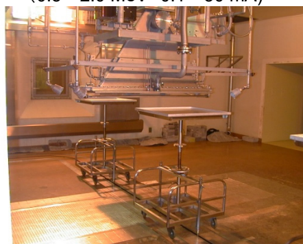
Electron irradiation room with conveyor system
