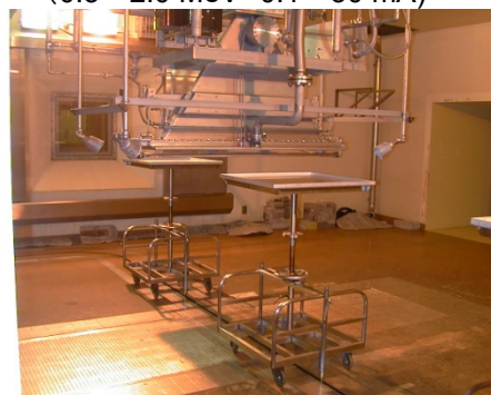
Electron irradiation room with conveyor system
