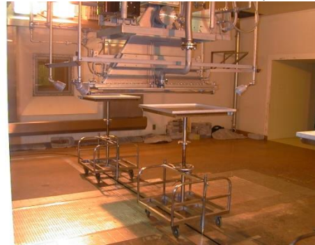
Electron irradiation room with conveyor system
